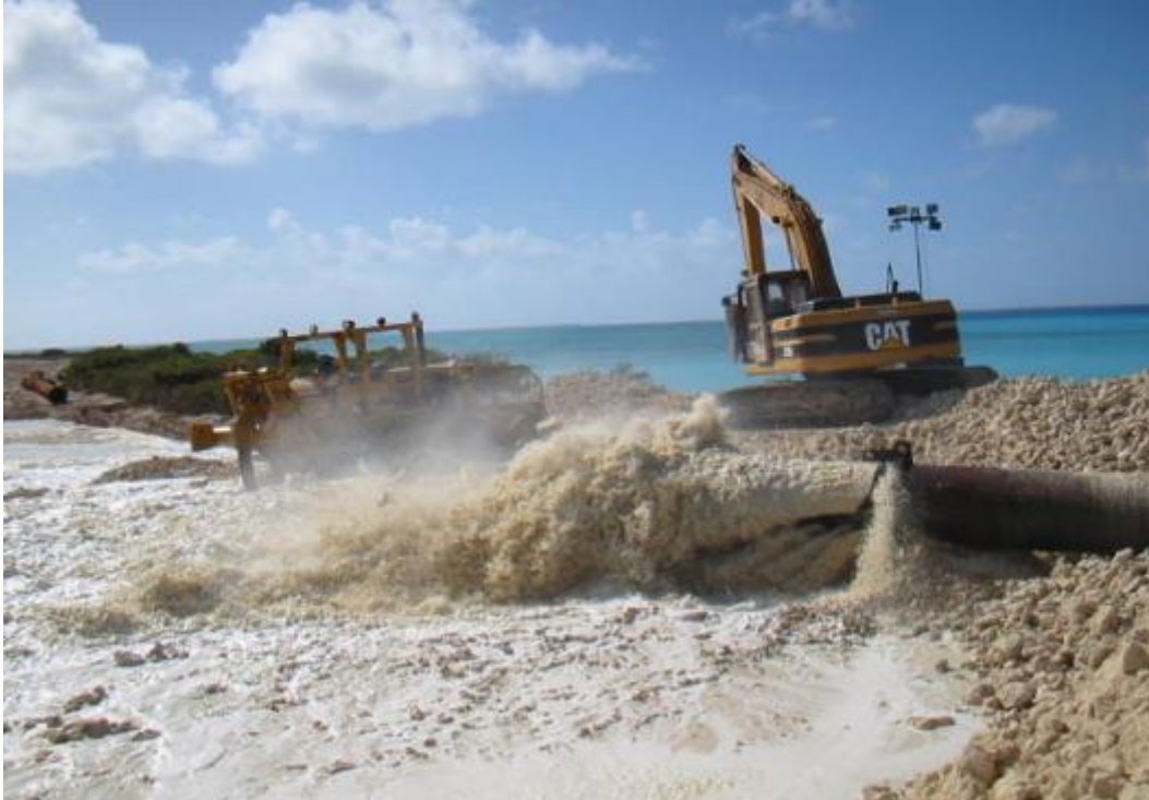
Photo 6.2. Representative photo of upland discharge of dredge material (Grand Turk Cruise Facility construction)
